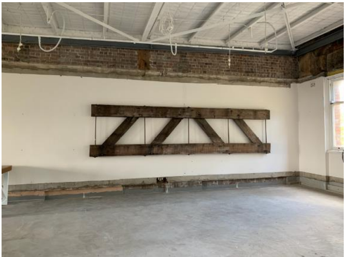
Figure 8: Evidence of original interiors within 74 and 76 Oxford Street and interpretive timber truss
